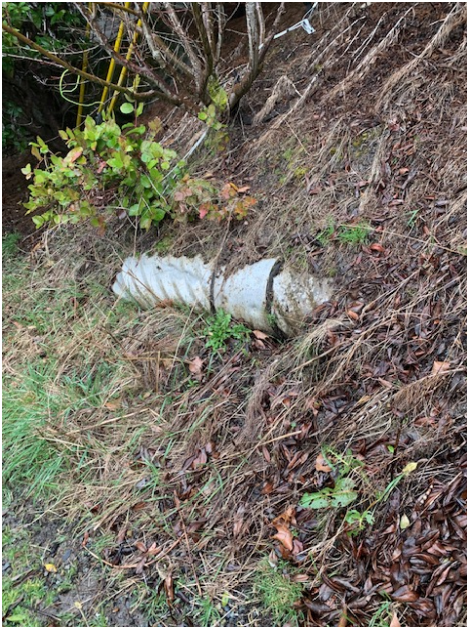
Exposed pipe next to trail near top of trail Point E, no joint leaking
