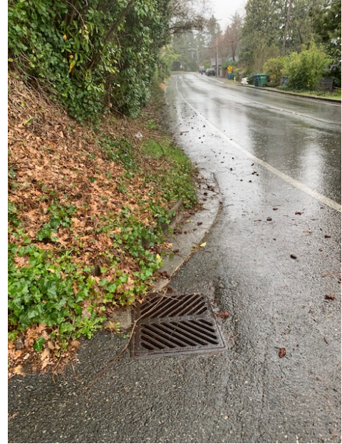
Catch Basin At Eath side of W Mercer Way, At Point L. End of Analysis Looking Downstream
