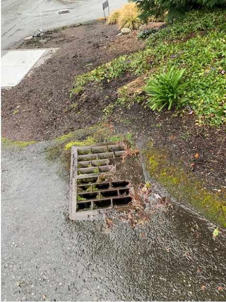
Catch Basin Point H - West of 69 th Ave SE at intersection - Looking West
