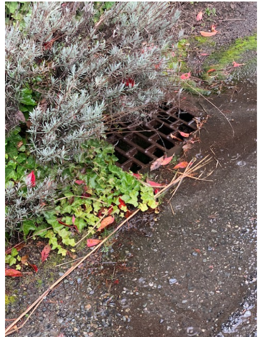
Near intersection East Edge Catch Basin – Point D
