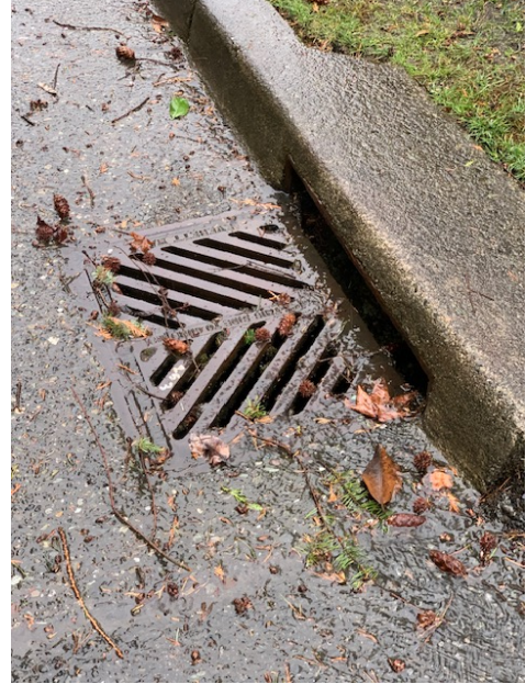
Catch Basin along Noth side of SE 32 nd Street, At Point I
